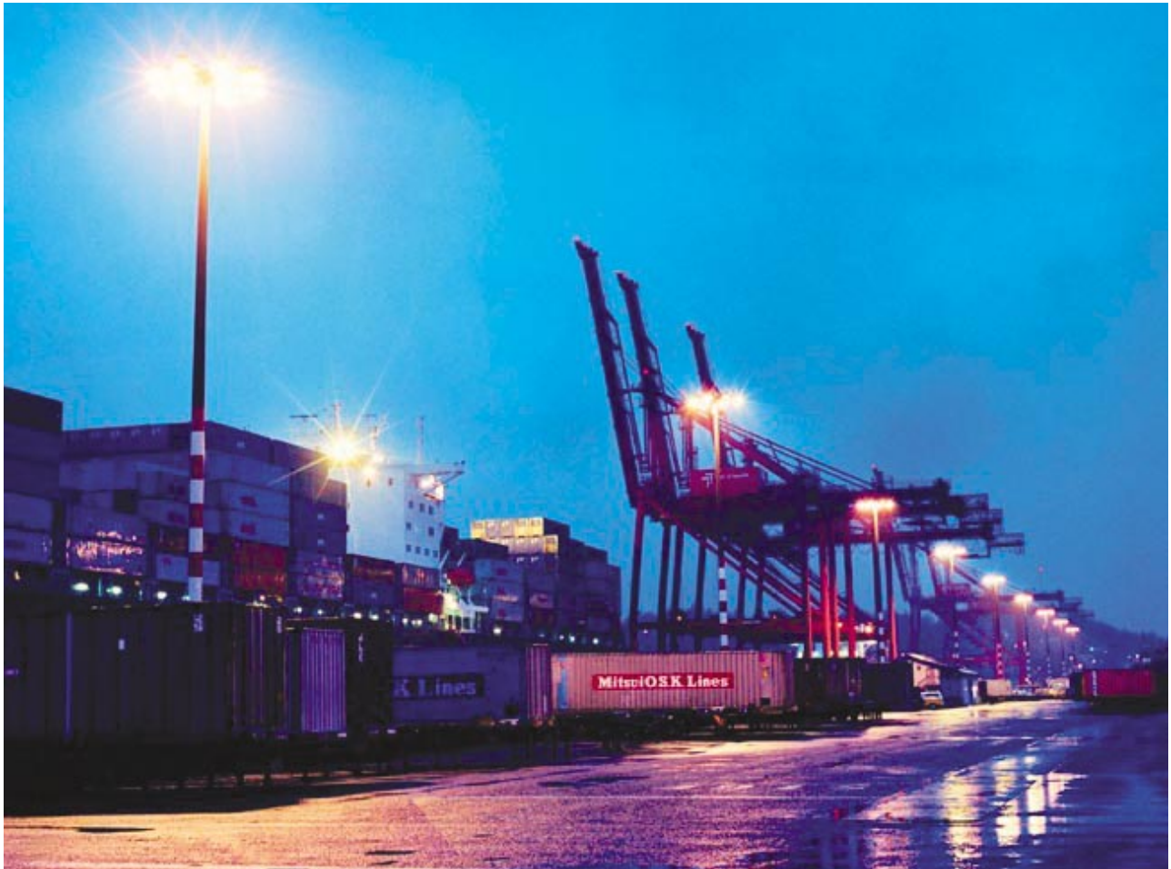
Figure 12. Uniformly spaced poles and luminaires provide lighting at each crane assembly area in this cargo terminal. (Photo courtesy of Holophane.)
