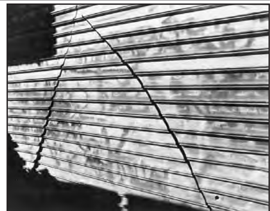
(Right) The top of the second cut is left unfinished until both sides are cut. Then, join the cuts. This allows the gate to stay in place during operations.
