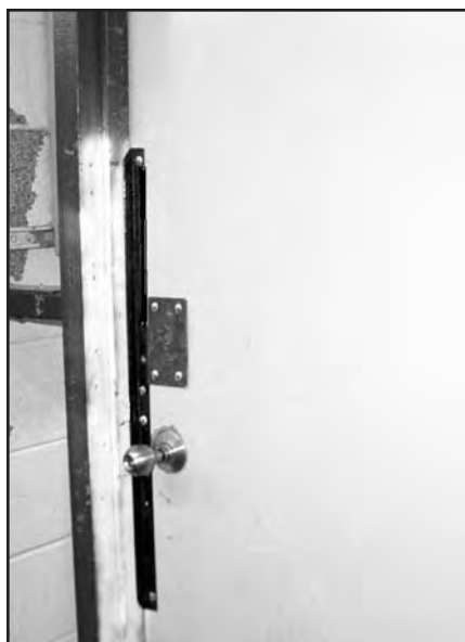
Figure #1--When performing forcible entry, Firefighters should use the angle iron to their advantage.
